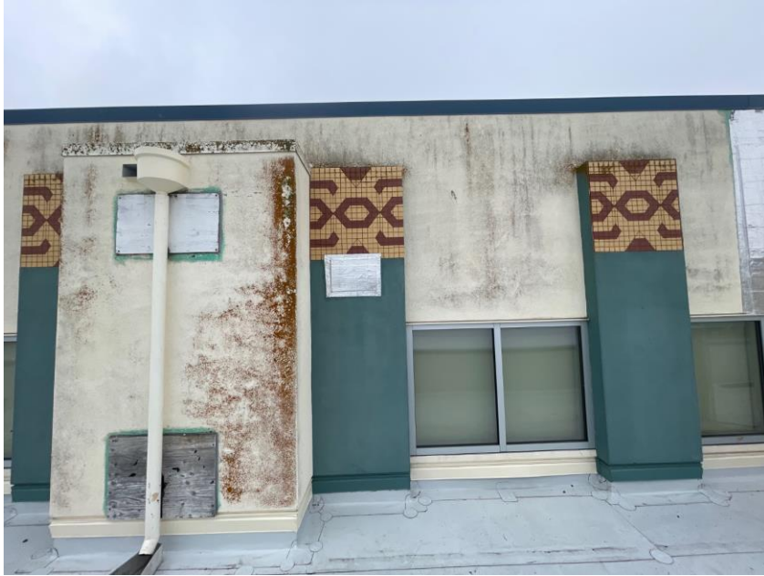
West Wall Before (with leaks)
